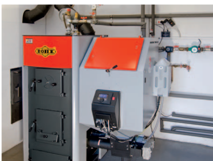
Model boiler room with boiler ROJEK TKA 25
